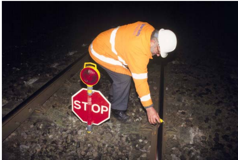
A track worker placing a detonator next to a possession limit board in accordance with Rule Book module T3 (section 5, clause 3: How to provide detonator protection).
